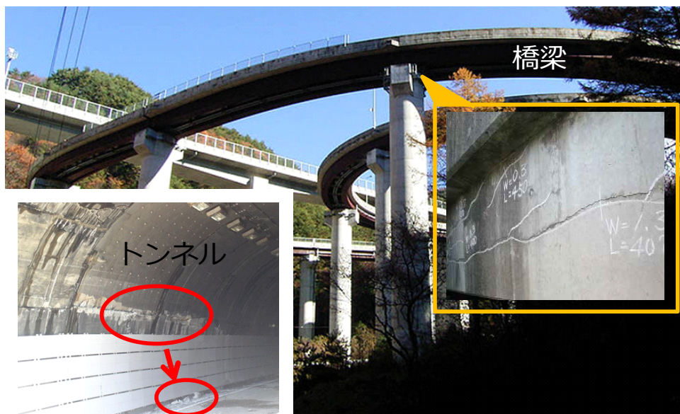
図 2.5: Images of bridges and tunnels: In Japan, there are more than 4000 tunnels that were built more than 40 years ago. Much is expected from flying robots for tunnel inspection work. However, it is a very difficult to measure “curved walls” with conventional flying robots.
