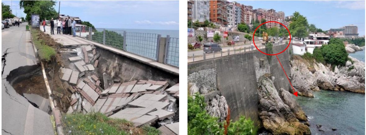
Figure 1 The Subsidence of Road and Sidewalk behind a Concrete Seawall in Zonguldak, Turkey (CNN TURK, June 25, 2015)
