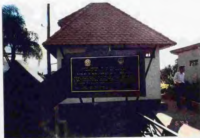
Photo 6. Effluent water monitoring house, which consisted of much monitoring equipments, by the technical cooperation of JICA for Brazilian Government in Santa Catalina.
