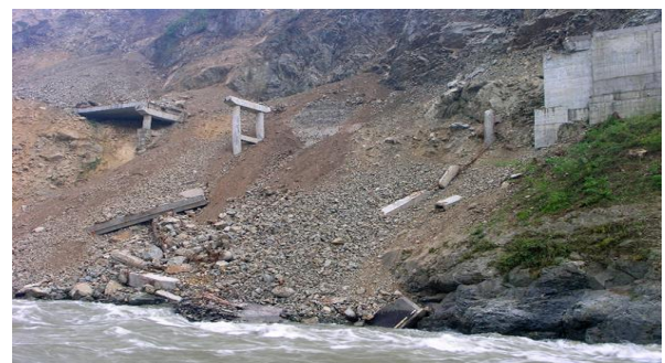
Figure 2. Damage to bridges due to landslides.
