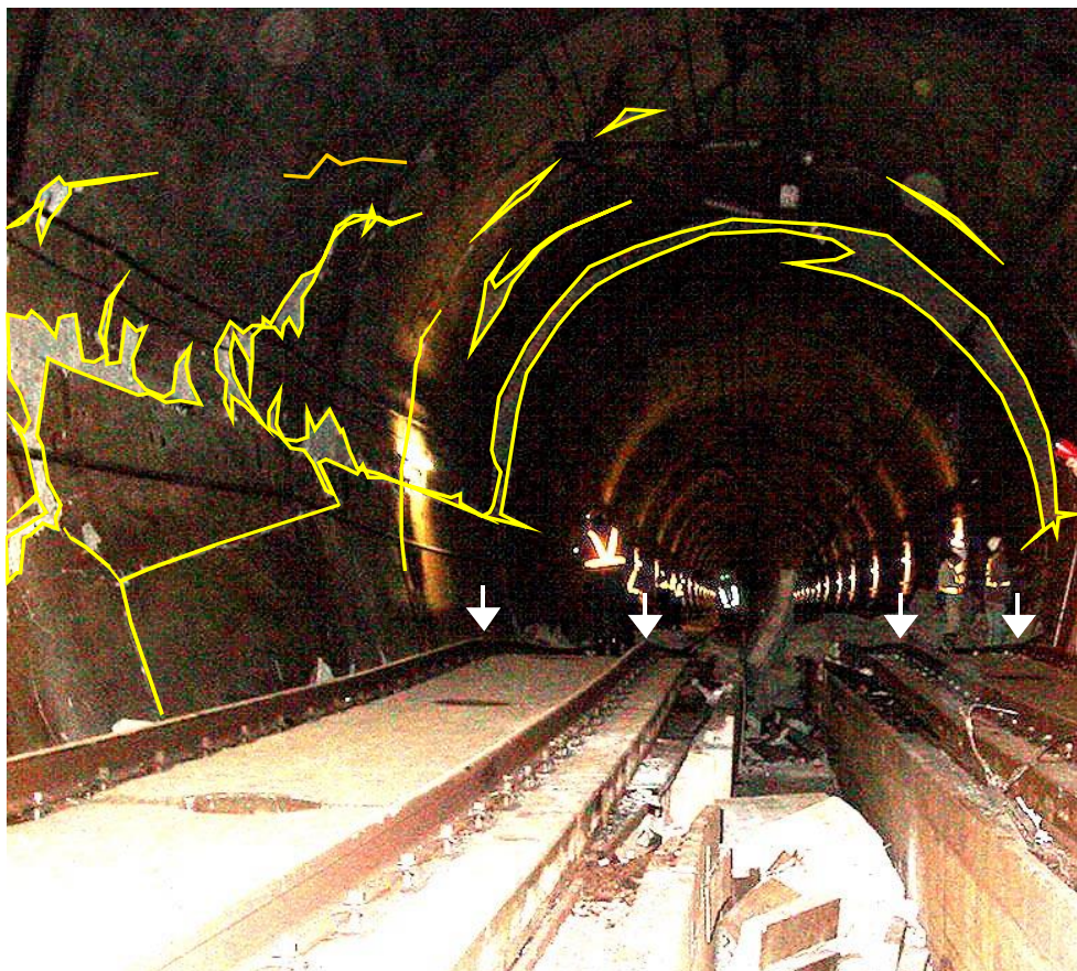
Figure 5.9: Most seriously damaged section of Uonuma Tunnel: The rail buckled together with the track-bed concrete slab, which was uplifted by about 250 mm over a 100 meters long stretch (see white arrows). A band of large cracks diagonally traversed the lining (yellow lines). Large concrete chunks fell down off the 5 m long section of the tunnel crown. Photo was taken at Point a_1 (37.2833°N, 138.86579°E), 195,050m from Tokyo Station by Konagai, K. (Johansson et al., 2007)
