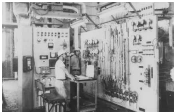
図 1.1 Old plant operation panel board(出典：[1])
