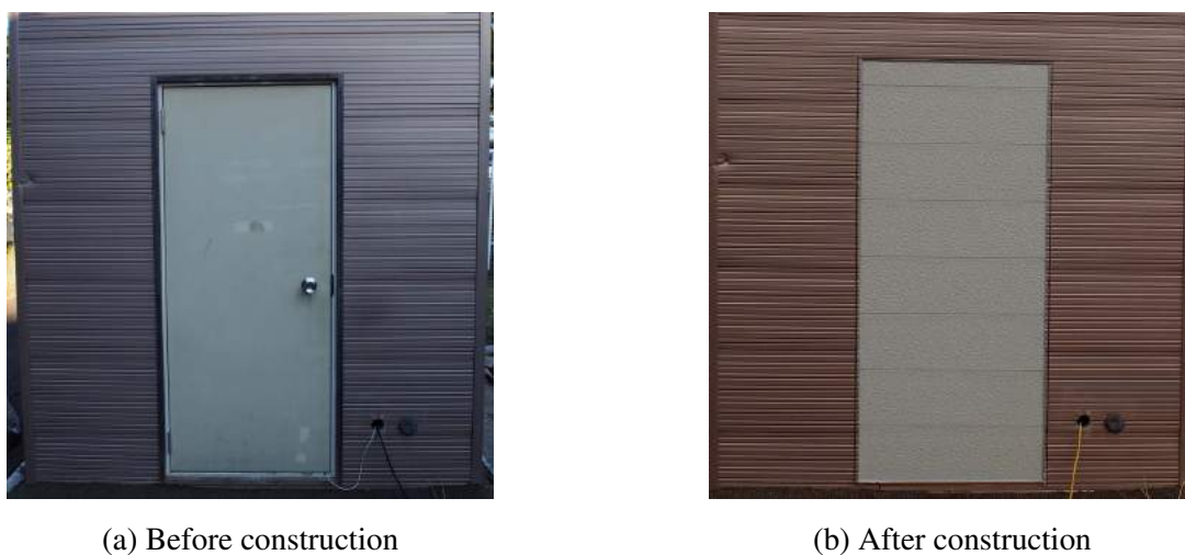
Fig. 4.9: Figure before and after the construction wall in the place where there was the door.
